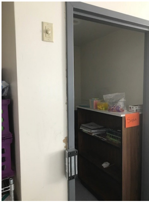
Former isolation room re-purposed into a storage room with no door.
